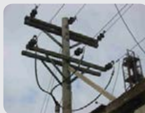
Distribution line faults
