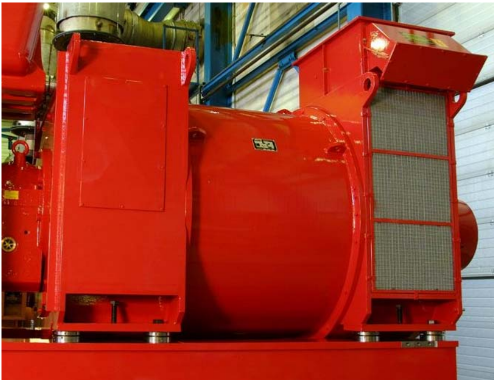
Figure 5.1.6.2 Generator of genset mounted on Vibracon ® chocks.
